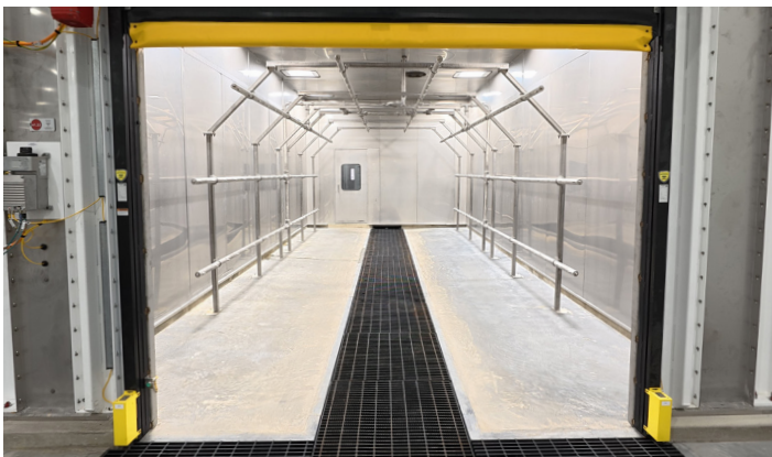
Engineered Wash Water Recovery Systems
